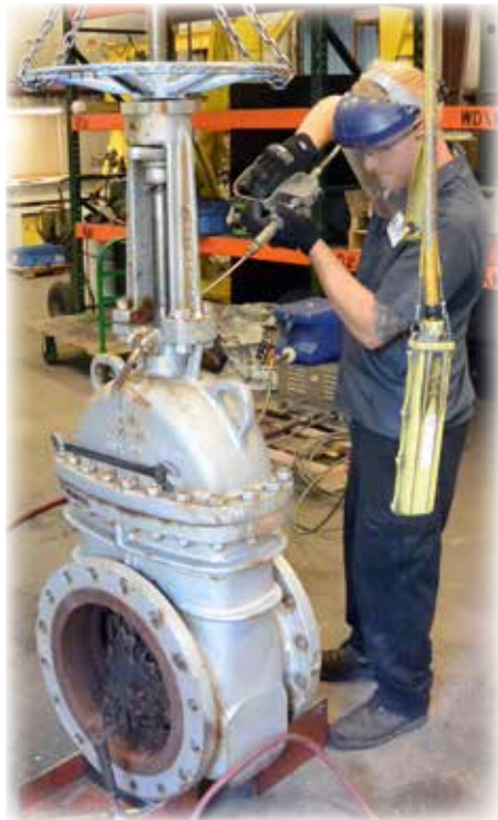
Technician extracts old packing from valve with special compressed air & liquid jet packing extractor.
