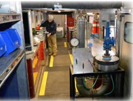
Interior view of the Mobile Valve Shop with valve technician at work in the fully equipped, self-sufficient, 53-foot trailer that visits customer sites for testing and repair.
